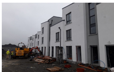
Construction at Pennefeather Green, Hebron Road. 3 bed duplex apartments, ground and first floor. 2 bed apartments on second floor. All own door units.
