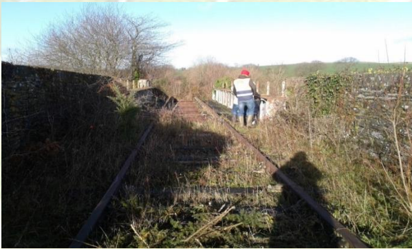
Examining one of the old bridge structures along the route of the South East Greenway at Carrickcloney.
