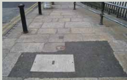
Temporary surface in a granite flagged footpath. Unfortunately it appears that several historic flags were removed or cut in the process of this installation and there has been no attempt made to design a cover appropriate to the historic location
