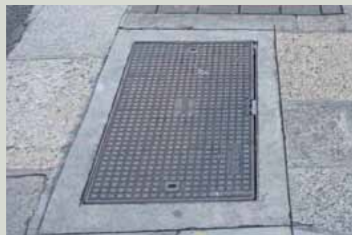
Poor workmanship and detailing: A wide border around the new insert has been backfilled with sand-cement mortar
