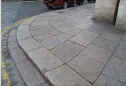
Stepped radial paving at Cork Hill, Dublin. The originally tooled slip-resistant surface has worn down to a smooth finish which exposes the buff-coloured structure of the granite adding richness to the visual quality of the street in particular when it is wet
