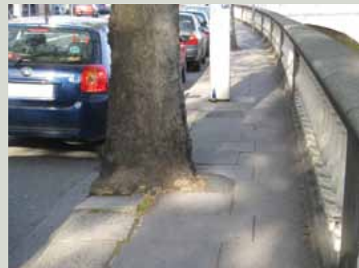
A lack of provision for the growth of the tree has led to damage and displacement of kerbstones and flags
