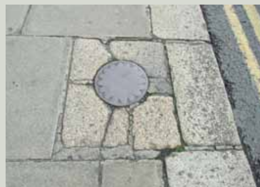
Damaged granite flagstone surround to a coalhole cover. However, despite the damage it should be retained in situ with whatever minor repairs are required to mitigate further damage
