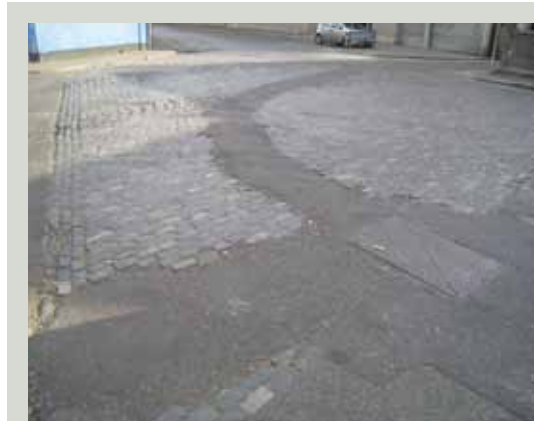
Extensive damage to a setted pavement caused by laying of underground services
