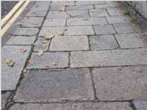
Slightly recessed joints allow the uneven edges of the historic flags to be seen which enriches the character of the paving. However, they have the disadvantages of catching dirt and small pieces of litter and allowing the accumulation of water which may make them unacceptable in some circumstances
