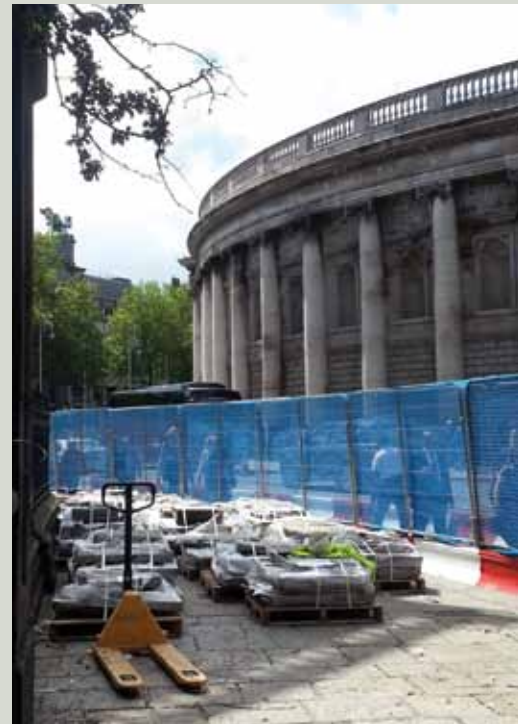
Lifted granite flagstones being prepared to be taken off site temporarily for storage
