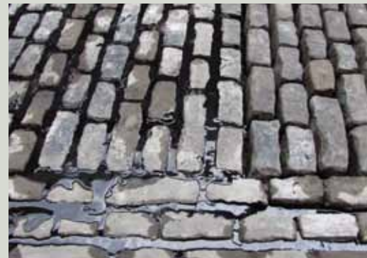
Untidy tar jointing allowing tar to run over the surface of setts
