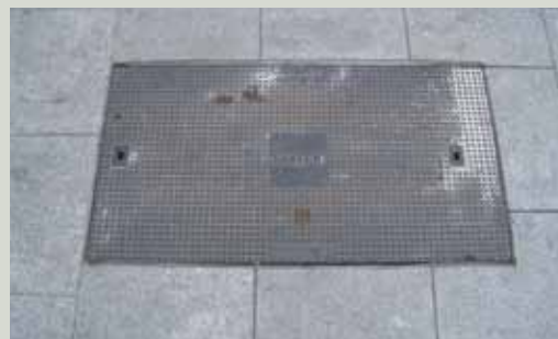
Good workmanship and detailing: new paving has been cut accurately around cover creating a tight joint and the cover has been placed parallel to paving joints
