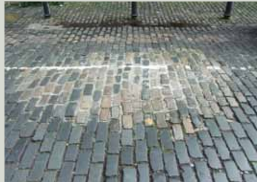
Unsuccessful repair using setts of different stone types, poorly set out and using inappropriate jointing material and methods
