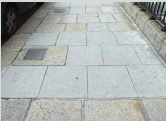
Replacement flagstones of an even size have been used to match the historic ones. However, the colour match is poor and the appearance of the machine-made finish of the new flags is jarring
