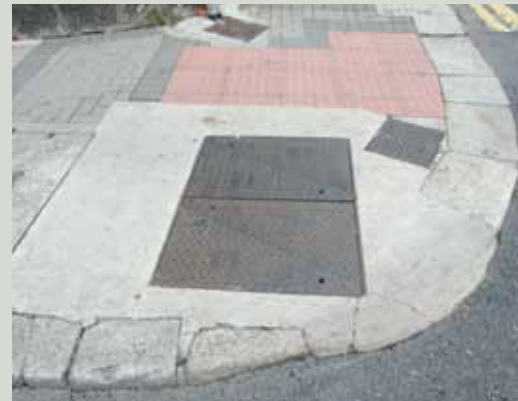
A series of uncoordinated works have taken place to this section of paving in a historic area resulting in the localised loss of the original paving and some kerbstones and an unsatisfactory patchwork of different materials. In addition, the position of the large metal cover at the corner has made it impossible to reinstate all of the granite kerbstones
