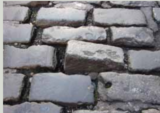
Failure of interlocking due to heavy traffic and lack of maintenance of joints causes unravelling of a surface
