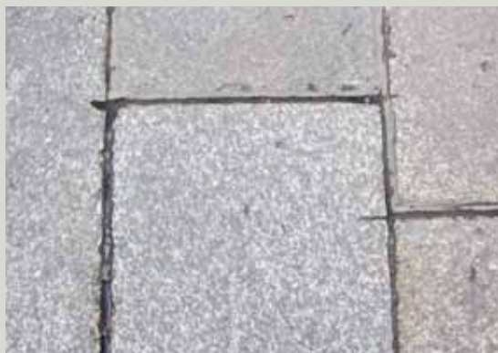
The use of power tools such as angle grinders should not be permitted in areas of historic paving. In this example, inexpert use has resulted in irreversible damage to the granite flags
