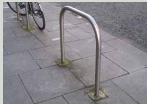
Bad detail: modern slabs which were cut after laying and poorly backfilled resulting in some flagstones cracking and others cut with power tools
