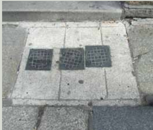
Access points set in concrete within a granite pavement in a manner not appropriate to the high-quality historic environment
