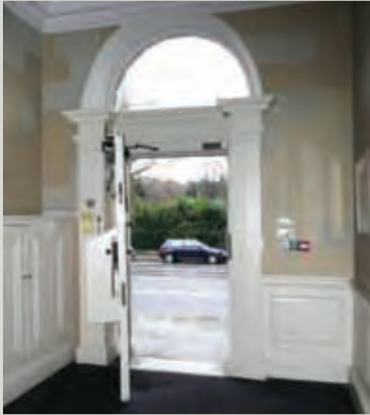
The addition of an automatic door opener on this heavy Georgian door has benefited everyone
