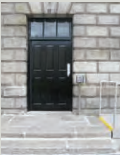
When carrying out the alterations to raise the landing and provide wheelchair access to this building the existing outward opening double doors which had been fitted in the 1980s were removed and a single new door and fanlight based on the design of a pre-existing door nearby was installed, thereby providing sufficient space at landing level for a chair to turn. An important consideration was the relationship of the new landing level to the door frame and other elements of the façade
